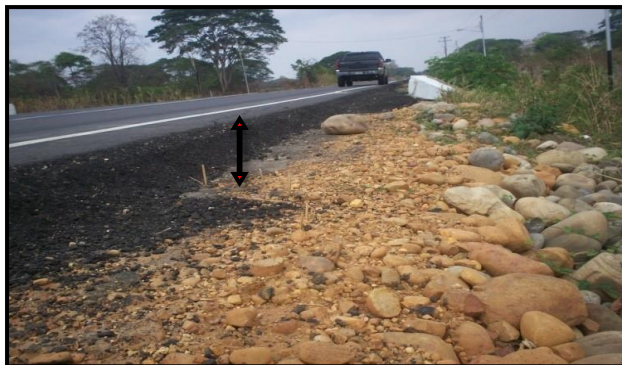
Figura 28: Desnivel – carril berma
